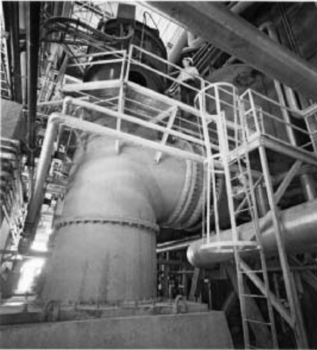
FIGURE 112 Vertical propeller pump installed (Flowsolve Corporation)
