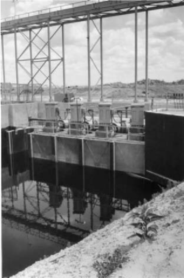
FIGURE 9 24 in (610 mm) discharge, 1250 HP (750 kW) vertical pumps (Hazleton Pumps, Inc.)
