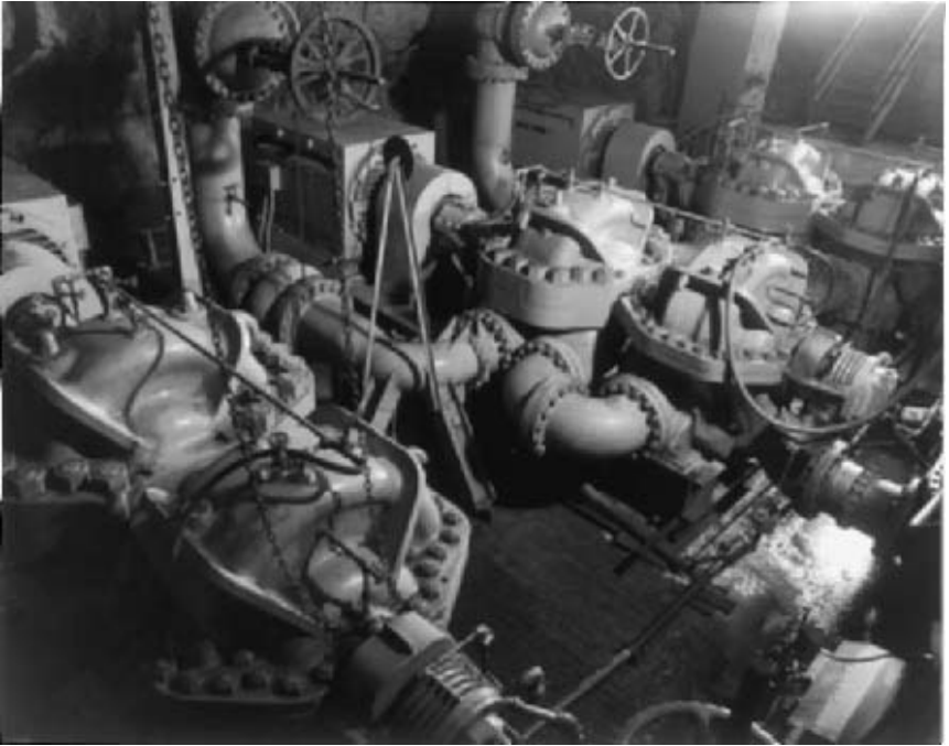
FIGURE 14 Three 2000 HP (1490 kW) pumps in one room in a zinc mine (Hazleton Pumps, Inc.)
