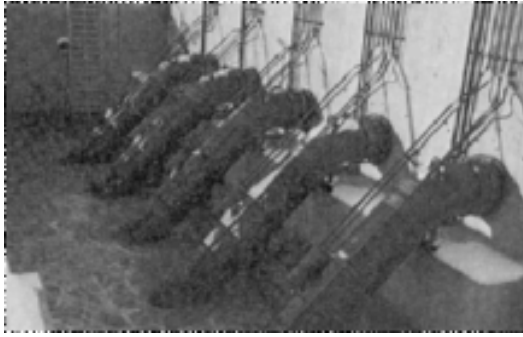
FIGURE 7 Five 42-in (107-cm) double-staged hydraulically driven water pumps with design flows automatically varying from 0 to 50,000 gpm (0 to 11,550 m 3 /h) (M & W Pump)
