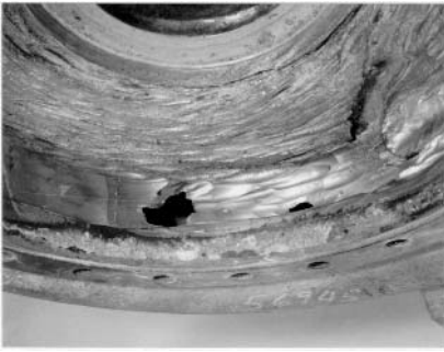
FIGURE 11 The severe erosion of a carbon steel casing in a 17% bauxite and sand service. Note the gouging due to the local turbulence of the slurry.
